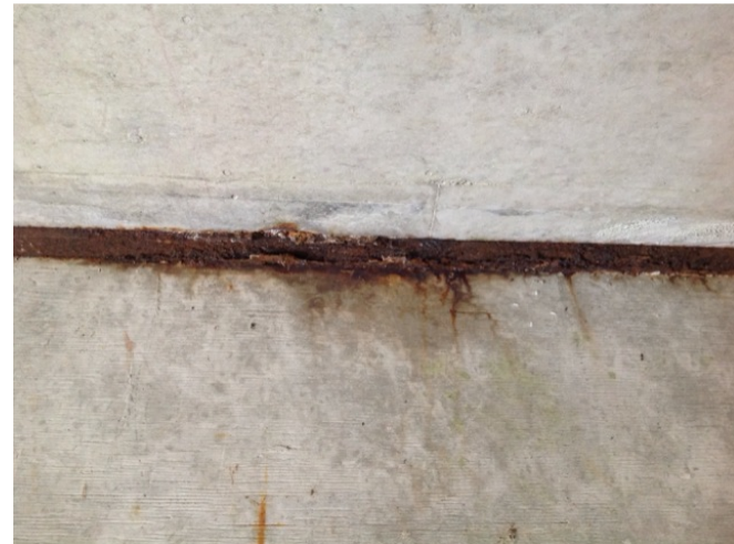
rusting girder at grout pockets
